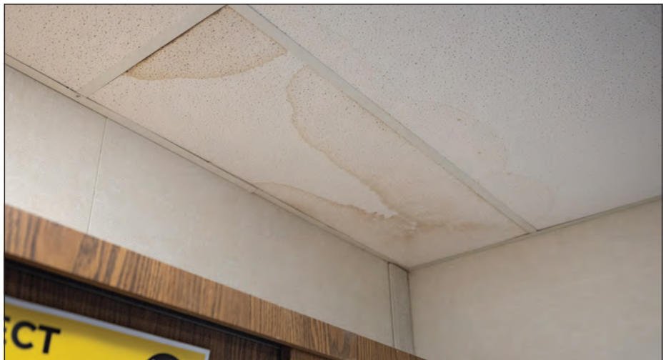
The structures have also been damaged after the unusually strong rainstorms of the past winter.
