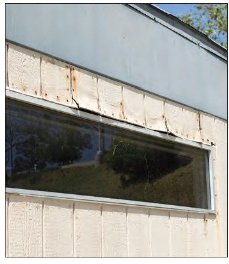
After serving as classrooms and meeting space for 30 years, the portable buildings are no longer safe.
